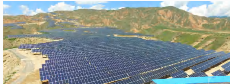
GCL SI Assisted in Building Hualong Rural Power Station and Contributed to Rural Revitalization
