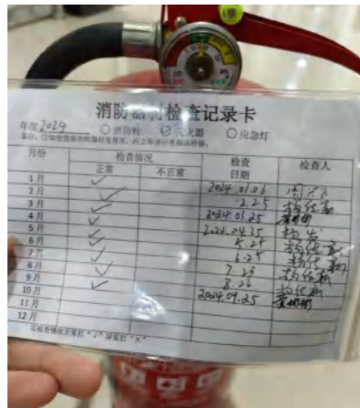
Monthly Inspection of Fire Extinguishers at GCL ET
